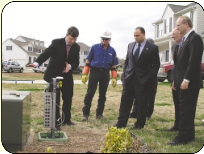
Amperion's Phillip Hunt shows FCC Chairman Michael Powell the hardware inside the ground-mounted pedestal.
