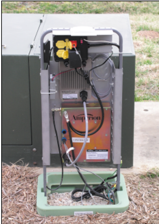
Inside the BPL “extractor,” the broadband signals are taken off the power line and fed to a “Wi-Fi” antenna for final transmission into subscribers’ homes. Amperion uses Wi-Fi for this last leg; other companies take the signal all the way into each house on the power line.
